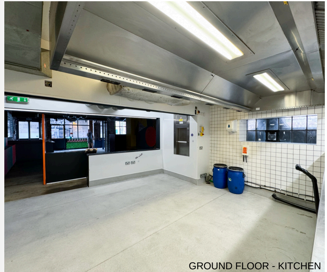
LOWER GROUND FLOOR - KITCHEN / REFRIGERATION
