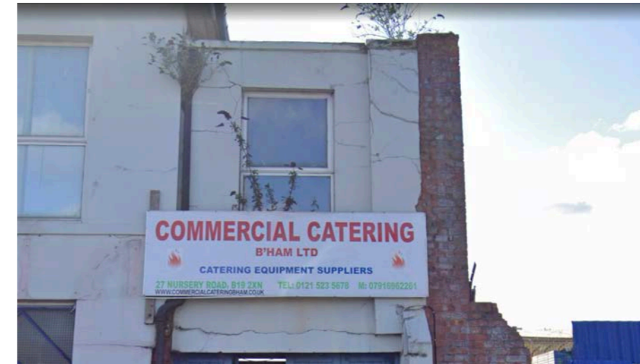
Visible cracking and deterioration
