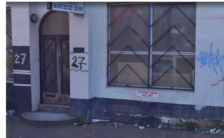
Vandalism / graffiti with unsightly window & door protection.
