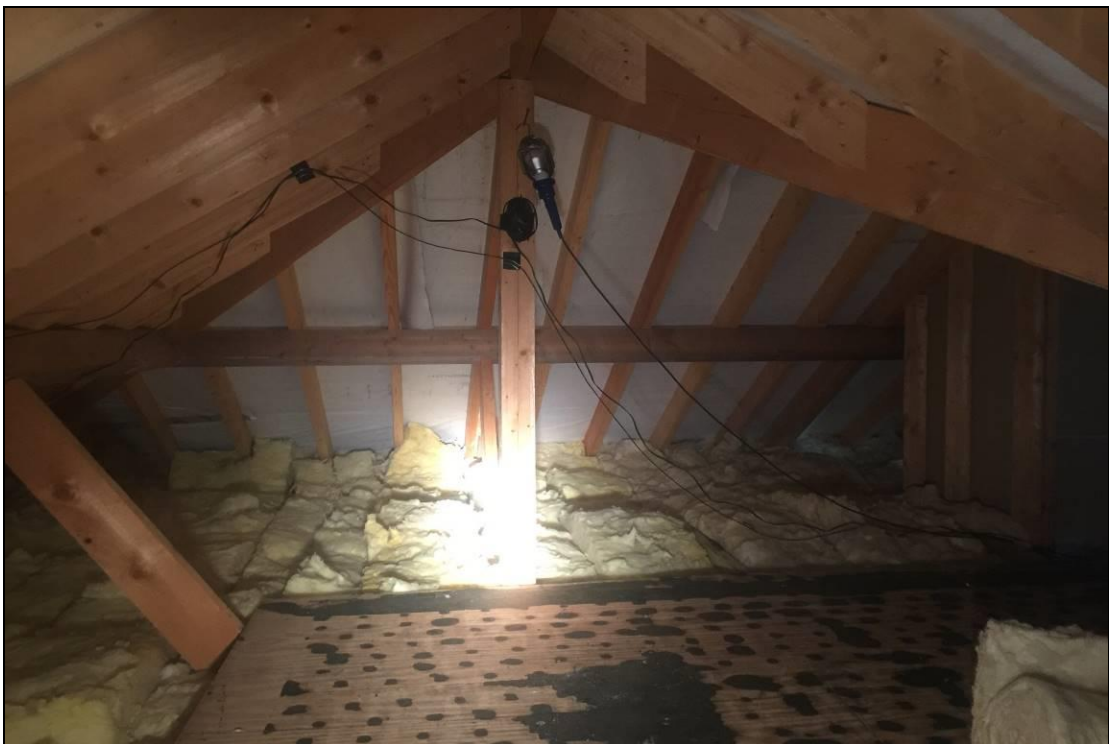
Photo 15: A more recent extension to the loft. This area is darker (although two Velux windows have potential to provide some light at the eastern end). The space is Tyvek lined. Again fibreglass is installed to the eaves, although minimal trussing is of value to eg Long-eared Bats, and there are a small number of features for crevice dwelling bats, including some missing mortar in-between breezeblock of the gable ends. However no evidence of bats was recorded and considered unlikely to support roosting bats in internal loft space.
