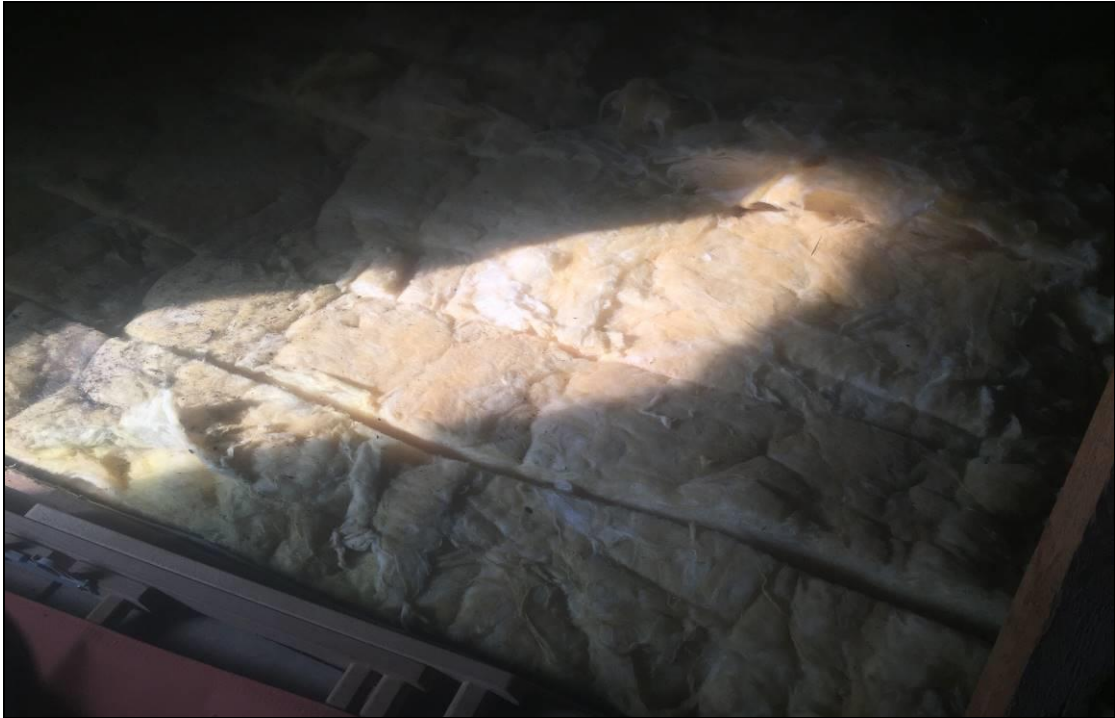
Photo 14: Loft well insulated with a double layer of fibreglass insulation installed against eaves reducing potential access points into the loft space.
