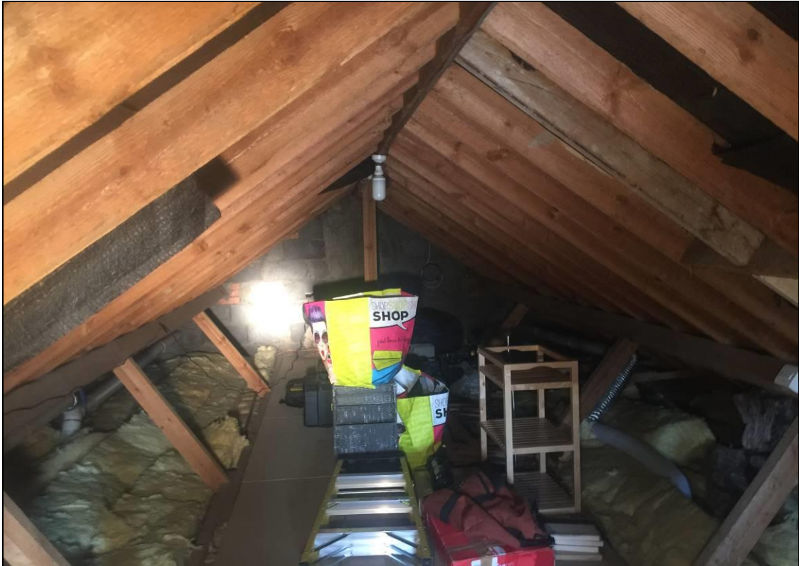
Photo 12: Internal main loft space. This is relatively light with a window at the southern end. The loft is bitumen lined. There was a small amount of light egress in a couple of areas suggesting access possibility (although upon inspection of the exterior this potential access point where light was entering was not identified). Overall no evidence of bats was recorded and considered unlikely to support roosting bats in the internal loft space.
