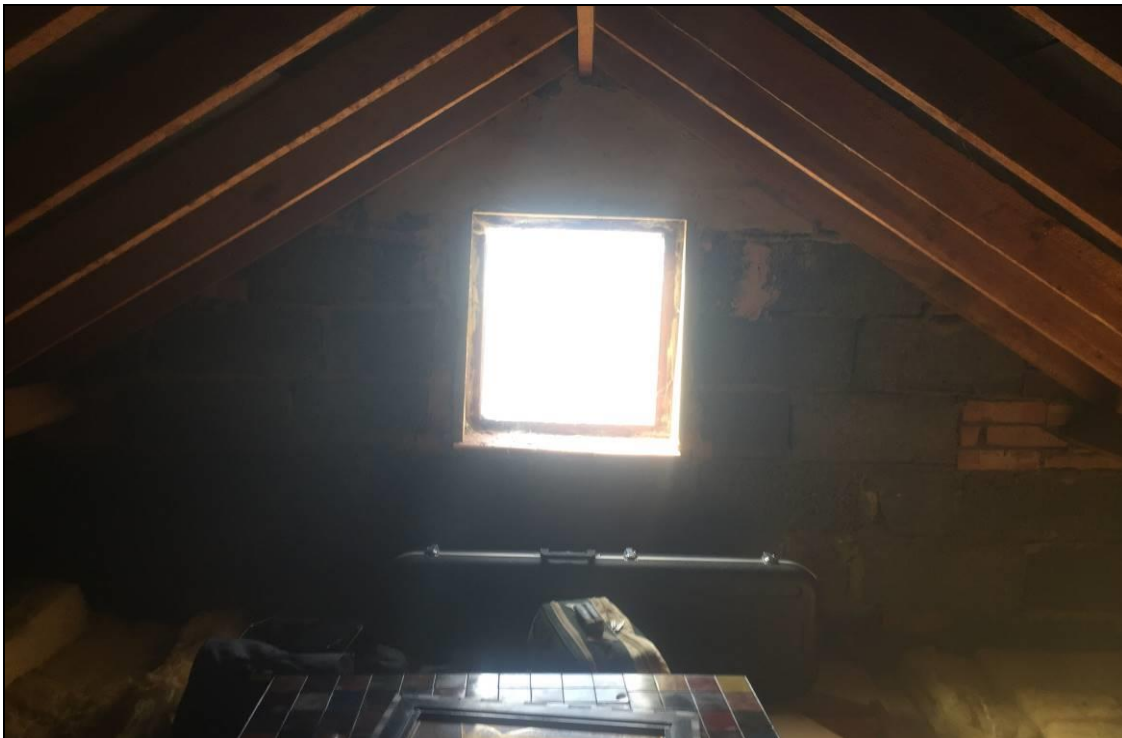
Photo 13: Window allowing light into main loft area reducing potential value to roosting bats
