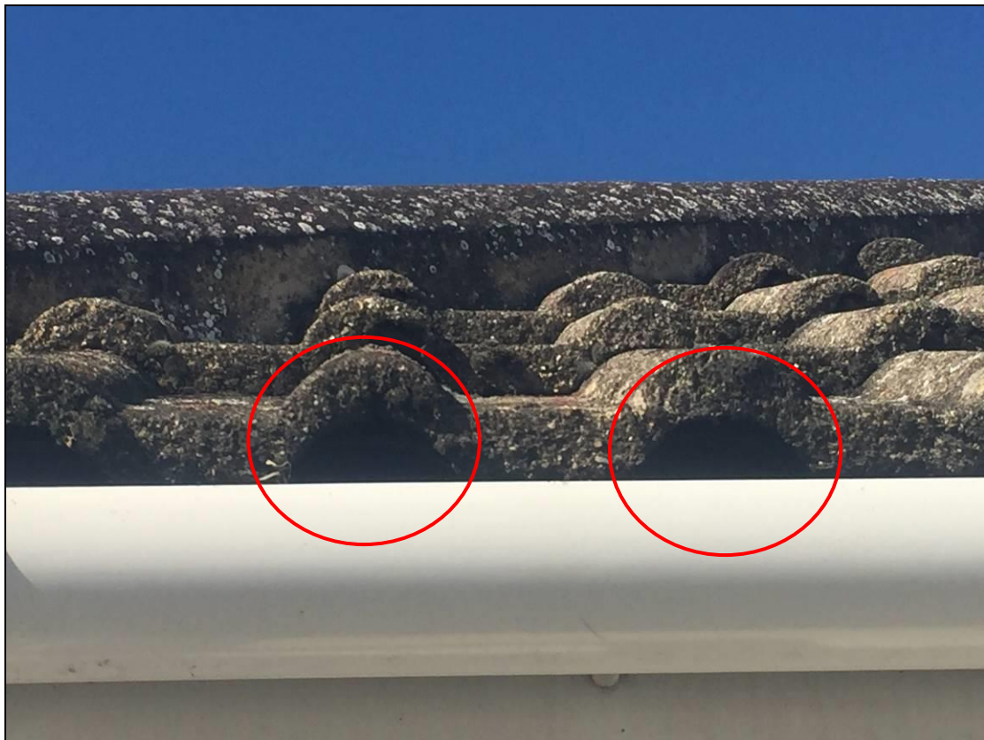
Photo 11: Externally the main bungalow has gaps of moderate-low potential at the bottom of the roof by the gutter. This is present on both front and rear of the property.
