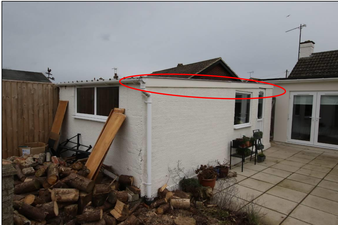
Photo 16: Bargeboards on garage contains small external gap with limited potential. Gaps could be inspected fully and no evidence of bats was noted. This gap is not considered to allow bat access into the interior of the building.
