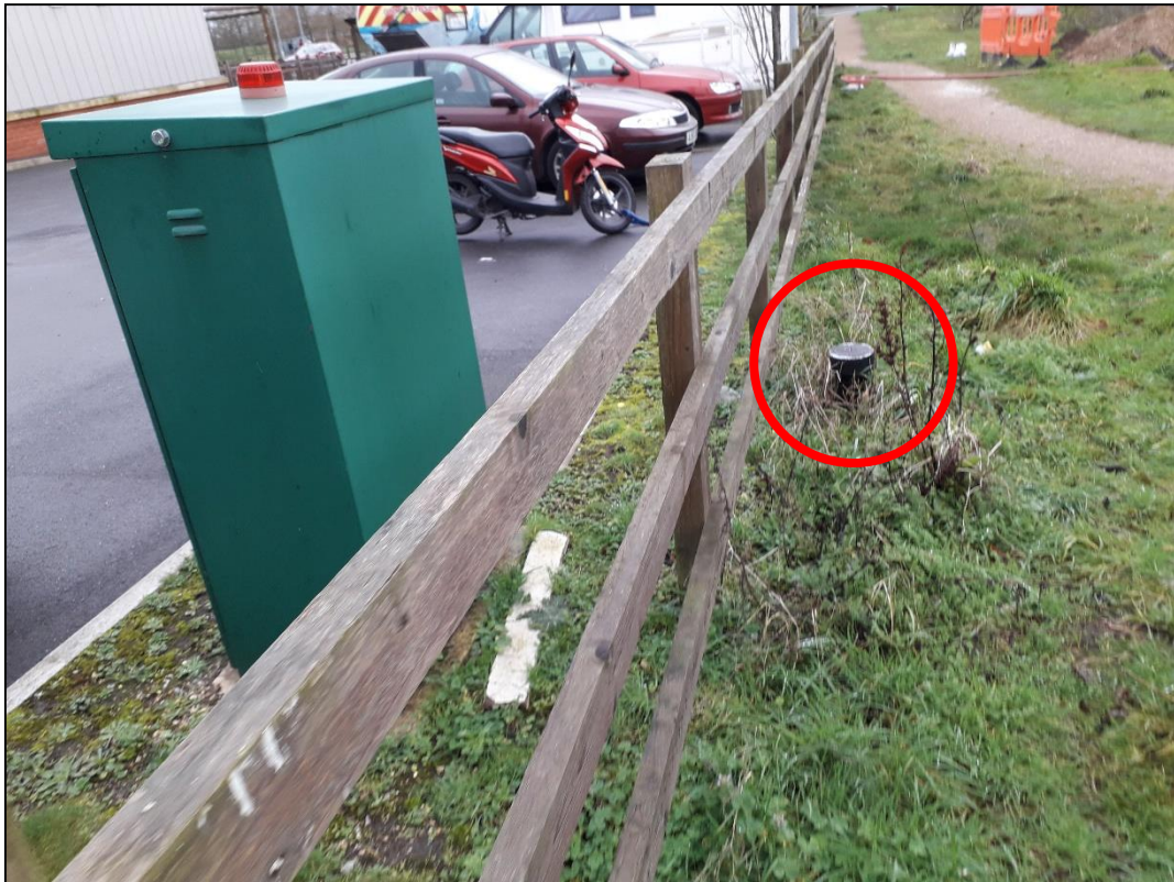
Gas vent pipe observed on eastern site boundary (view to south)
