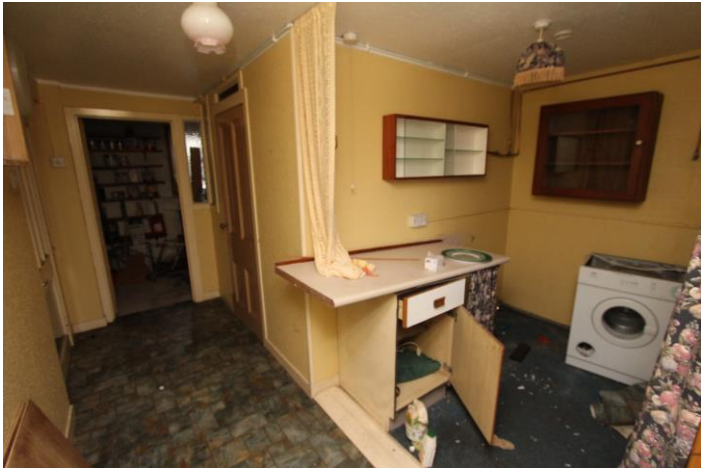
Basement flat utility room
