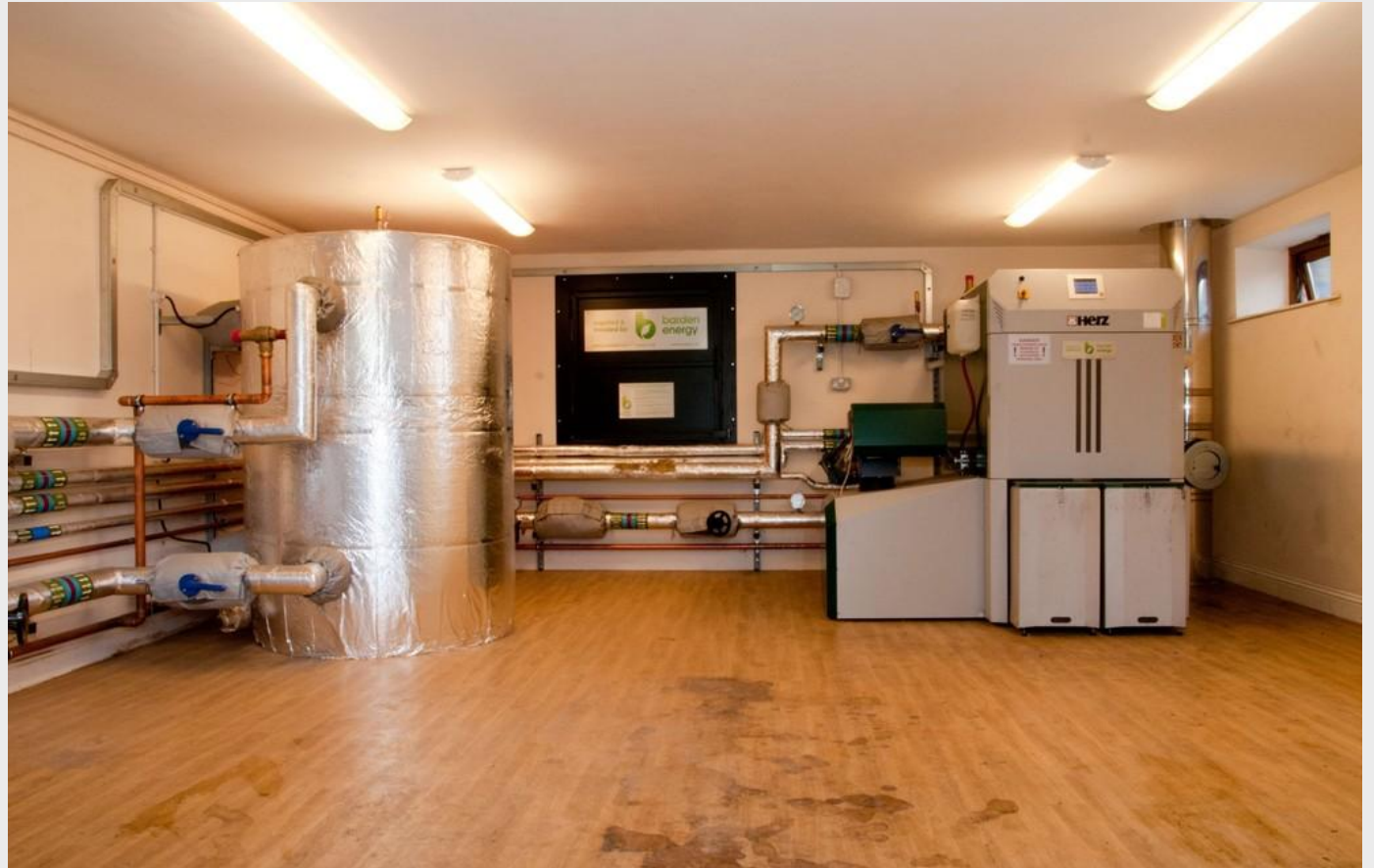
Heating Plant Room
