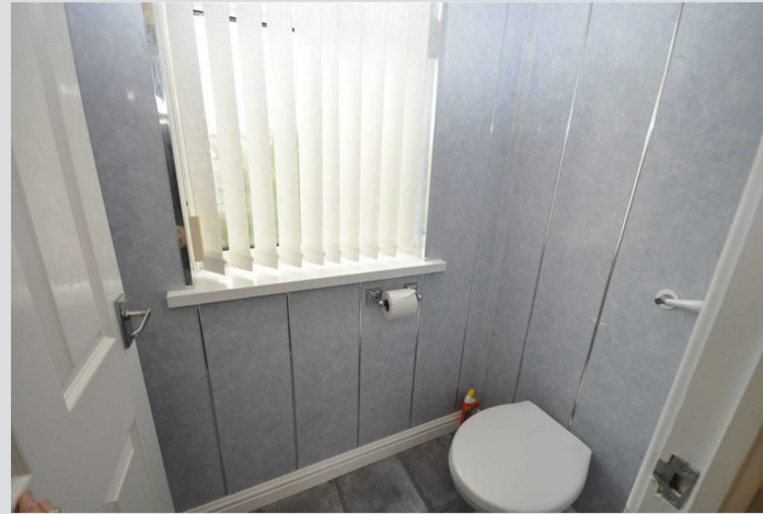
Low level WC, UPVC window to rear.
